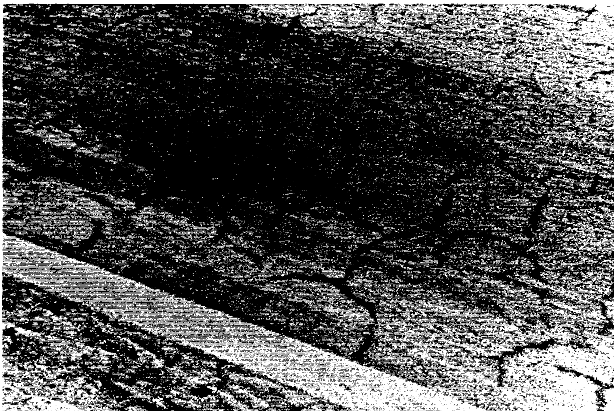
Figure 1. Fine pattern cracking on bridge deck.
