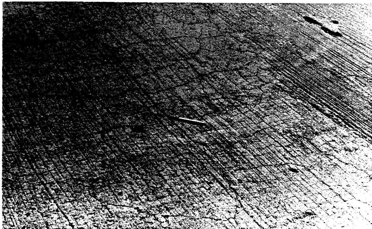
Figure 3. Transverse crack across roadway width.
