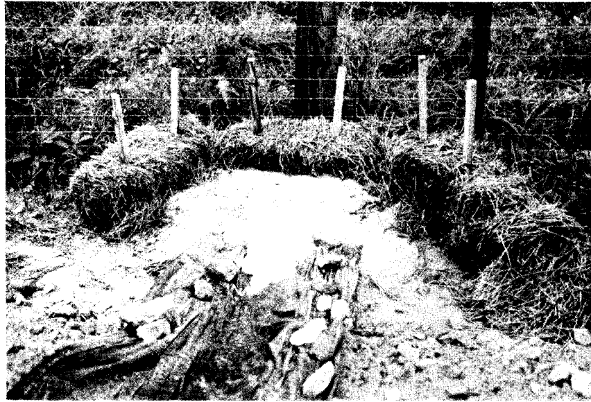
Figure 14. Silt transported by T-55 downdrain.
