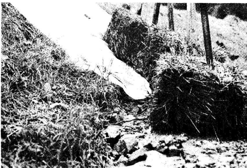
Figure 13. Undermining of torn polyethylene downdrain.
