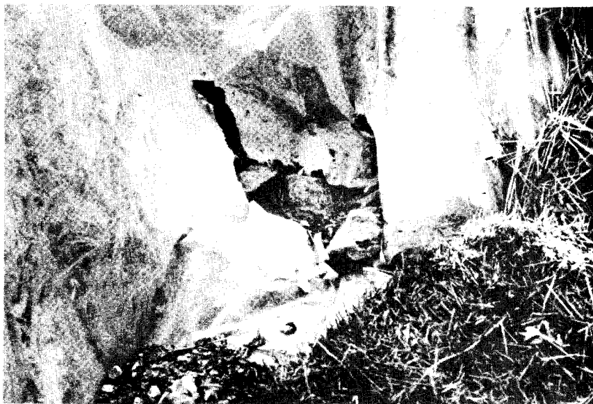
Figure 12. Tear in polyethylene downdrain.
