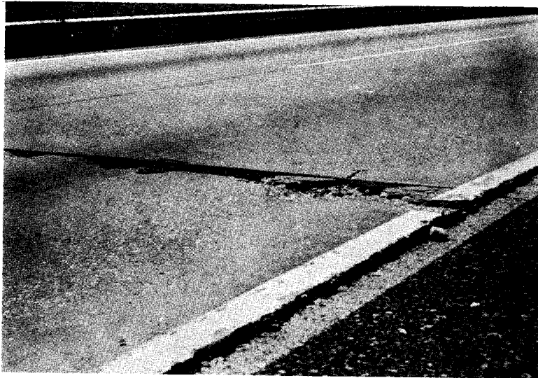
Figure 14. Joint crushing due to pavement pressures.
