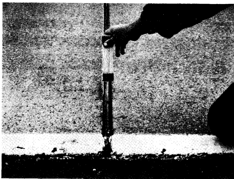
Figure 5. Excessive opening of joint near pressure relief joint. Note that the preformed seal is pulled away.
