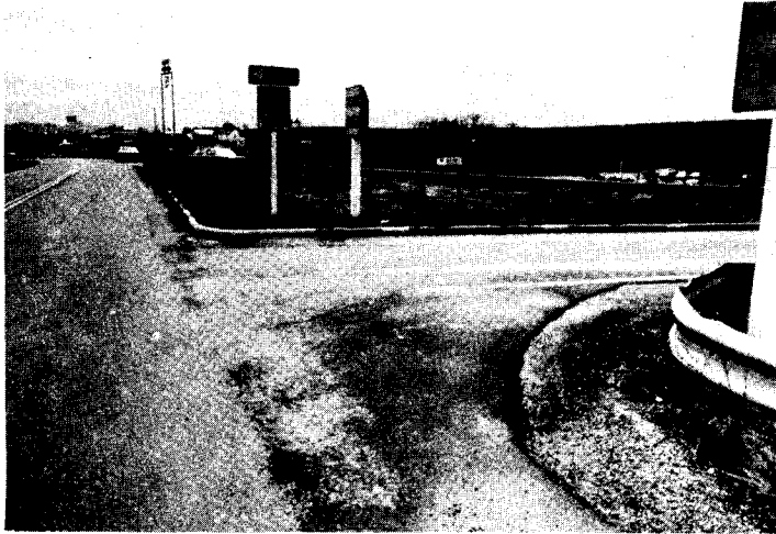
Figure 4(a). Present condition — view from crossroad of exit ramp where wrong-way entry took place.
