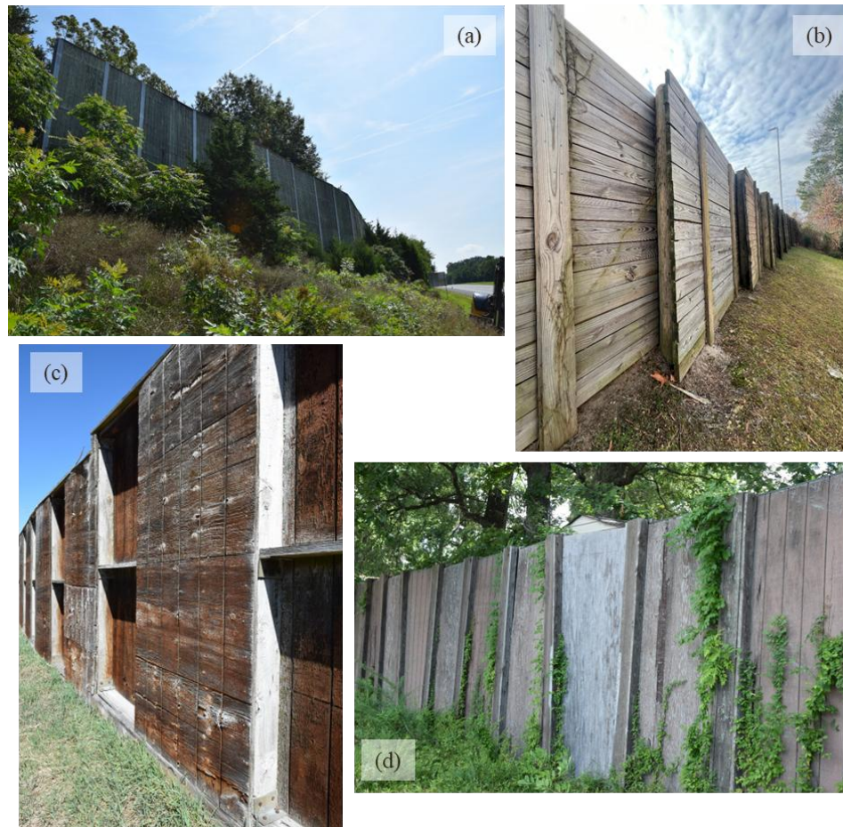
Figure 12. Photos of the Condition of Noise Barriers Constructed with Wood Panels: (a) Good Condition Noise Barrier with Metal Posts; (b) Good Condition Noise Barrier; (c) Old Noise Barrier in Good Condition; (d) Subpar Quality Wood Panel Noise Barrier in Poor Condition with Vegetation Growth and Flaking Wood
