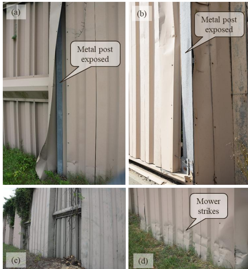
Figure 6. Additional Photos of the Condition of Noise Barriers Constructed with Metal Panels Oriented Vertically: (a) Impact Damage Leaving Metal Post Exposed on Ground-Mounted Barrier; (b) Impact Damage Leaving Metal Post Exposed on Bridge-Mounted Barrier; (c) Vegetation Growth; (d) Mower Impact Strikes on Ground-Mounted Barrier
