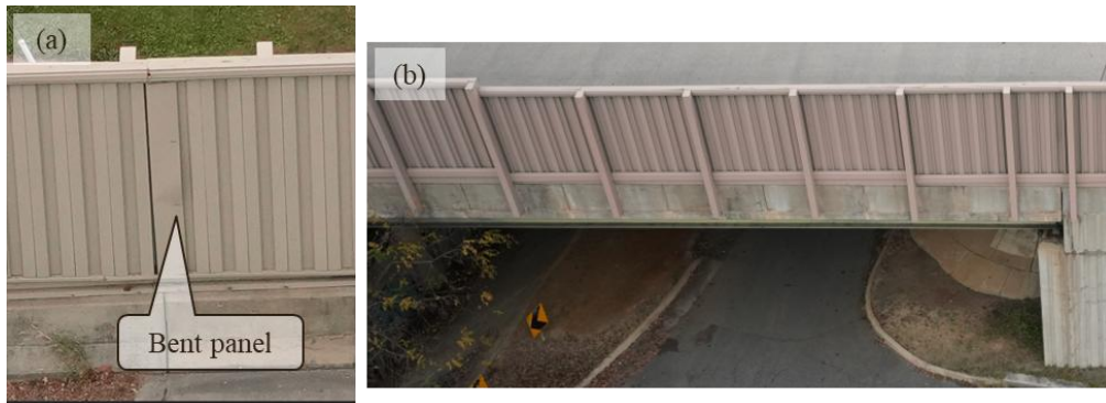
Figure 24. Screenshots from Colorized Mesh Model of Metal Noise Barrier at Fredericksburg Site: (a) Bent Panel on Front Side of Noise Barrier; (b) Back Side of Noise Barrier
