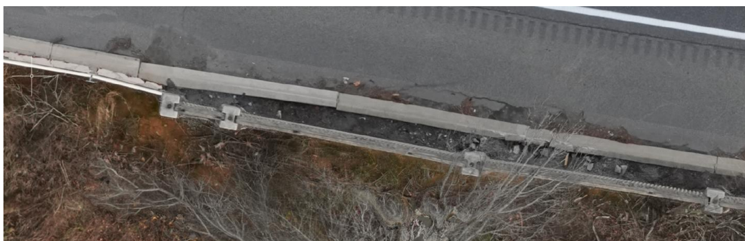
Figure 19. Orthomosaic “Top of Wall” Photo Where the Polyvinyl Chloride and Concrete Noise Barriers Join at Christiansburg Site
