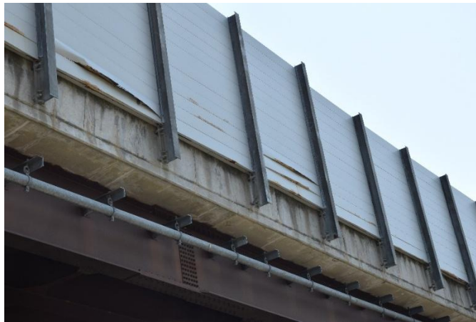
Figure 2. Example of Corrosion Damage on Metal Noise Barrier in Virginia
