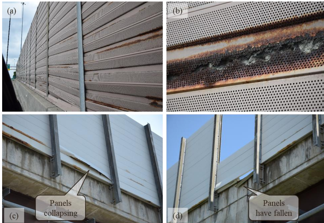
Figure 7. Photos of the Condition of Noise Barriers Constructed with Metal Panels Oriented Horizontally with Perforations: (a) Overall View from Roadway Side of Corrosion Present Throughout; (b) Closeup from Roadway Side of Corrosion Damage on Front Face of Panels; (c) Panels Collapsing Viewed from the Back Side; (d) Back Side View Showing Missing Panels that Have Fallen to the Ground
