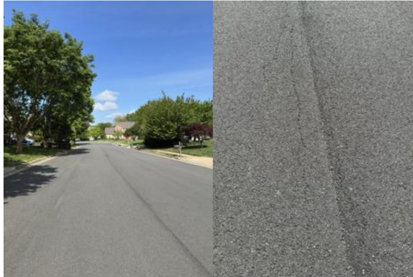
Figure 24. Images of Pavement Surface Condition on Walney Park Drive prior to Treatment
