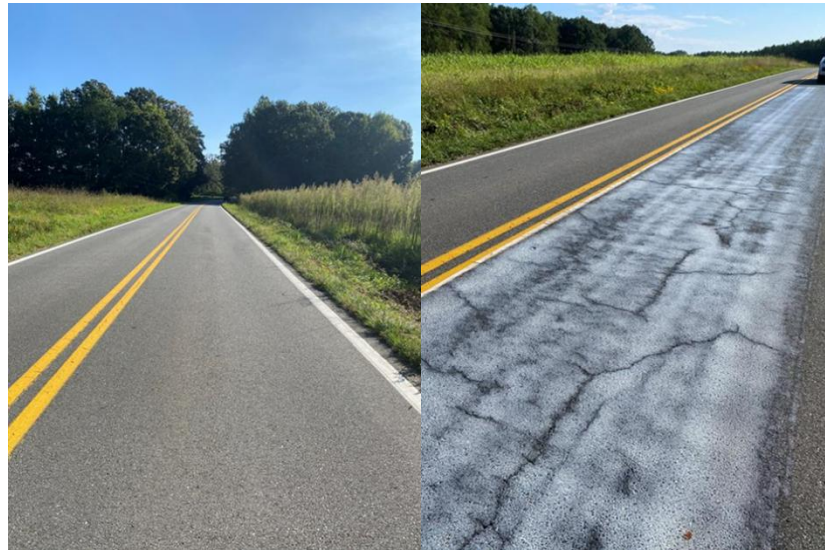
Figure 4. Images of Pavement Surface Condition on Route 640 with Areas of Good Condition and Localized Cracking
