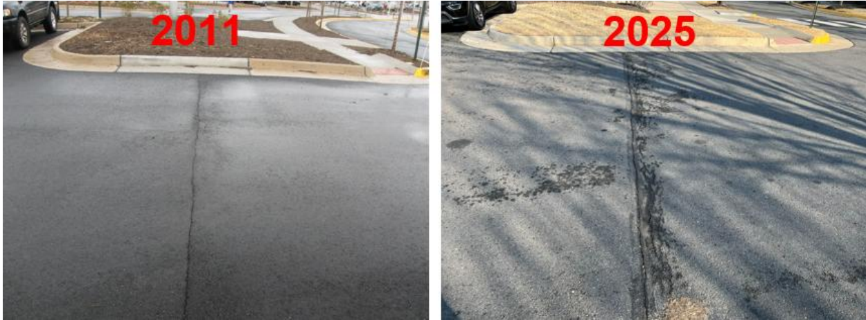
Figure 3. Surface Condition of a Northern Virginia District Parking Lot Prior to Spray-on Rejuvenator Application (2011) and during a Follow-up Site Visit in Late 2025. The spray-on rejuvenator was applied in 2016, followed by crack sealing. No additional surface treatments were applied between 2011 and 2025. Images provided by David Shiells of VDOT Northern Virginia District.
