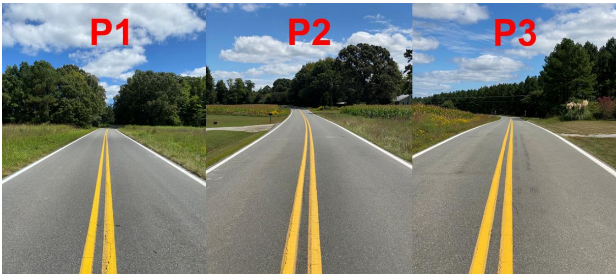
Figure 22. Images of Surface Appearance Approximately 12 Months after Spray-on Rejuvenator Application for Route 640. P1–P3 denote segments receiving spray-on rejuvenator application.
