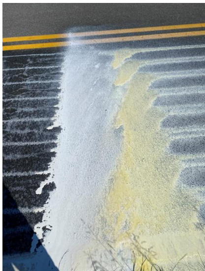
Figure 8. Localized Spill of Spray-on Rejuvenator Observed during Application
