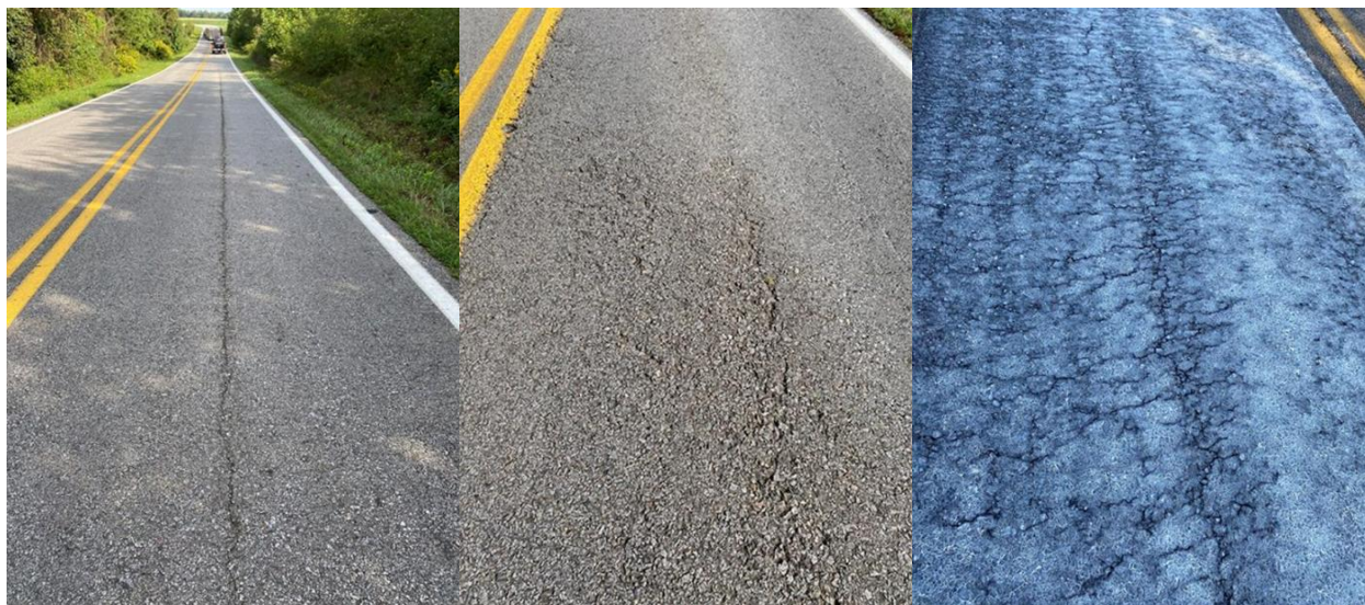
Figure 5. Images of Pavement Surface Condition on Route 750 with Areas of Cracking, Raveling, and Interconnected Surface Distress
