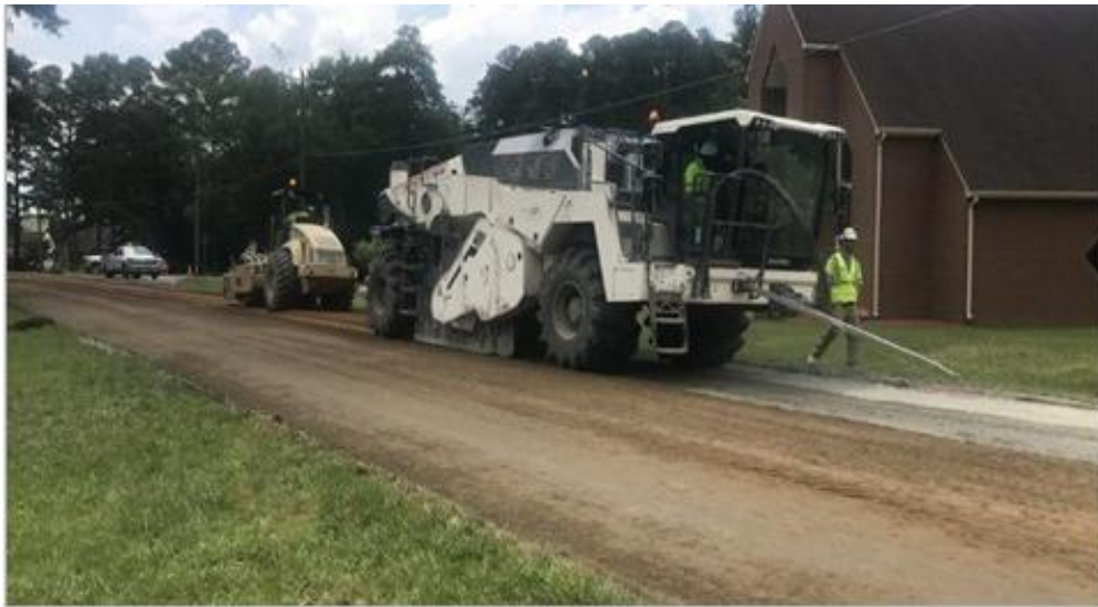
Figure 5. Conventional Full-Depth Reclamation Project on Route 216 Guinea Road in Gloucester County, Fredericksburg
