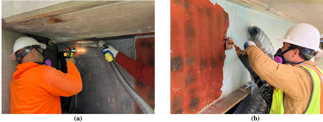
Figure 21. Fume Extraction Issues with LACR and ICR. (a) Employees observed using the effiSCAN LACR with the fume extraction nozzle removed; (b) The ICR unit was not equipped with any fume extraction, and workers were observed holding a 12-inch flexible duct near the work area in an attempt to capture dust and fume. ICR = induction coating removal; LACR = laser ablation coating removal.
