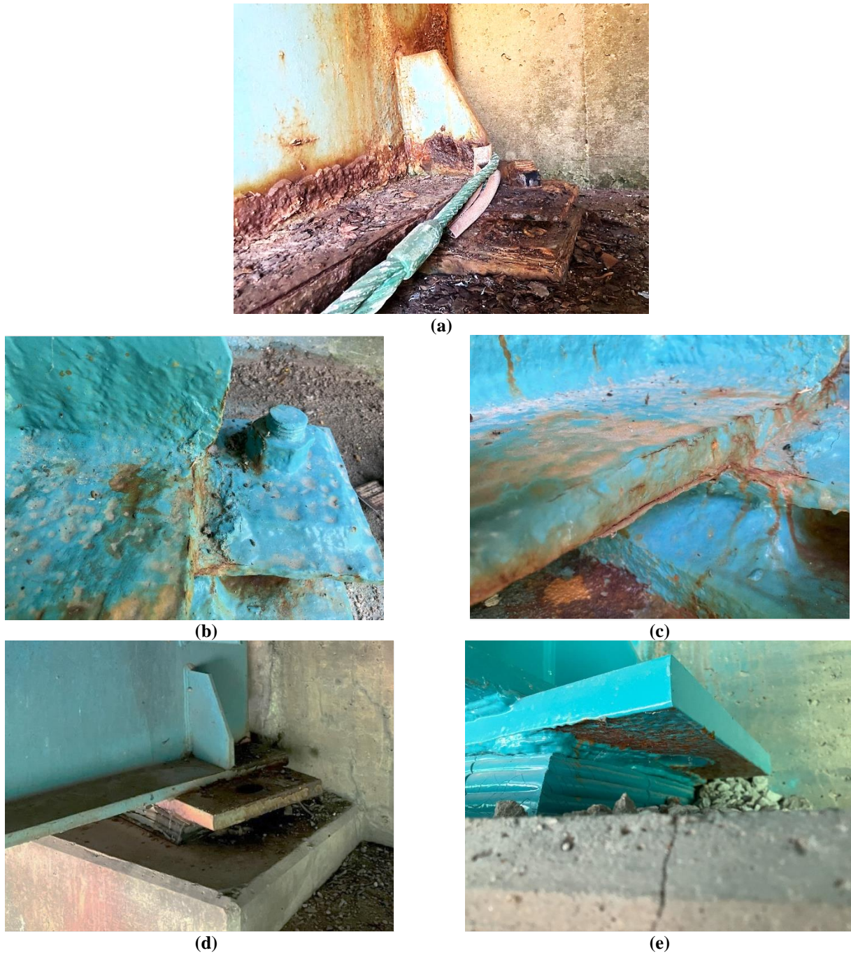
Figure 24. South Abutment A Girder No. 1: (a) Before Coating Removal, Showing a Cable Anchored above the Bearing for Abrasive Blast Cleaning by the Induction Coating Removal and Laser Ablation Coating Removal Specialty Subcontractor; (b and c) The Cable Passes between the Bolt and Stiffener before Recoating, Creating Difficulties Accessing this Area and Resulting in Rusting; (d) North Abutment B Girder No. 4 Bridge Bearing before and (e) after Abrasive Blast and Recoating Showing Rusting under the Plate due to Difficulties Accessing this Area.
