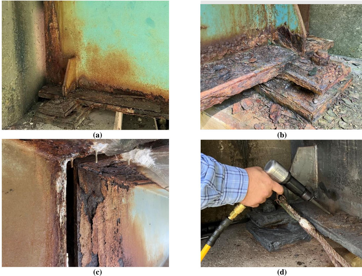
Figure 20. Rust Products on Bridge Girders and Bearings Result in Several Types of Corrosion, Including Lamellar and Pack Rust Formations, Often due to Leaking Bridge Joints. (a) Before coating removal, the web and bottom flange, plus the bearing, exhibit corrosion attack that is voluminous in nature. (b) Loose rust product and more adherent product are shown on the bearing, bottom flange, and web. (c) A more lamellar corrosion behavior is seen along the upper part of the web and the top flange. (d) Removing this product, which can be tightly adherent, can require mechanical removal, which is shown in this case using a pneumatic chisel breaking off the more tightly adherent product that must be removed to ensure salts (chlorides) are exposed and removed before performing a final cleaning step with Laser Ablation Coating Removal.
