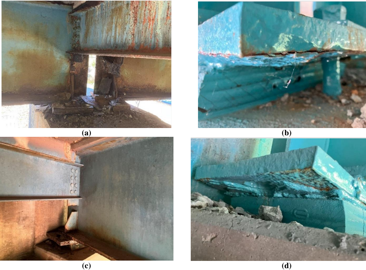
Figure 25. Pier 1 Girder No. 1 Interior: (a) Showing Pack Rust Under Sole Plate before ICR+LACR and then (b) after Sufficiently Cleaning Most of the Bearing Area with ICR+LACR but Leaving Some of the Pack Rust on the Bottom of the Sole Plate; (c) Abutment B Girder No. 4 Bridge Bearing before Abrasive Blast Cleaning and (d) also Showing Incomplete Removal of Pack Rust, Resulting in the Salt Initiating Corrosion Again. ICR = induction coating removal; LACR = laser ablation coating removal.
