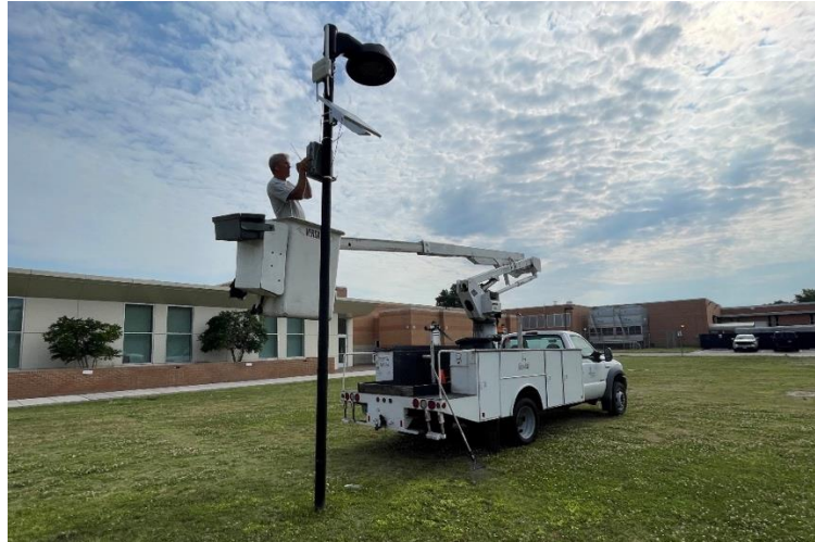
Figure 10. ODU Facility Management Staff Assisting in the Installation of a LoRaWAN Gateway, Solar Panel, and Battery Enclosure
