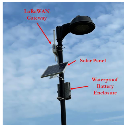
Figure 11. The Installed LoRaWAN System Mounted on a Light Pole
