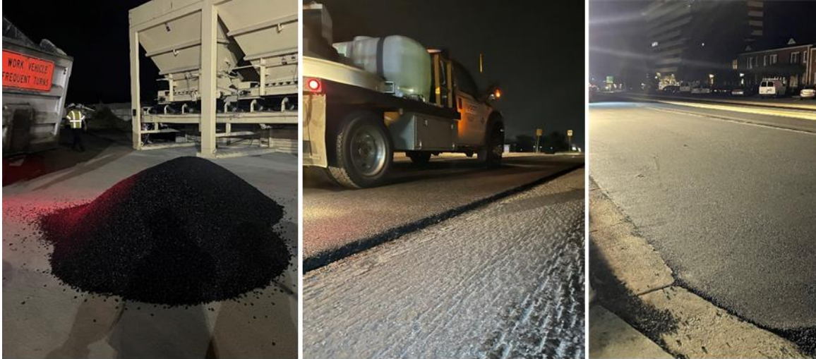
Figure 1. Production Operations at the Plant and Paving/Construction in the Field for HRMA and Reference Mixtures. HRMA = hybrid rubber modified asphalt.
