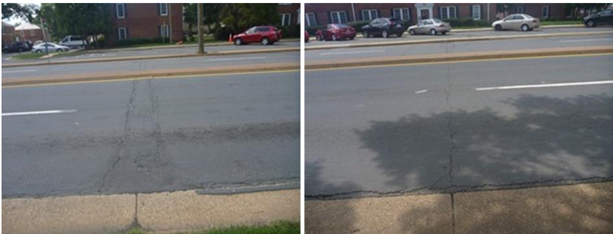
Figure 3. Reflective Cracking on the Route 120 / Glebe Road Existing Pavement Section
