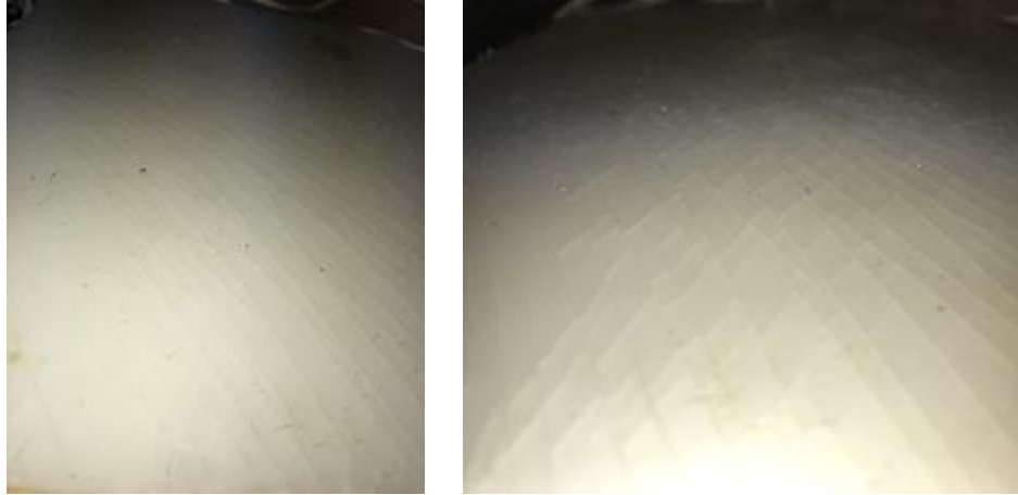
Figure 22. Superficial cracks on the interior side of an old high-density polyethylene plate
