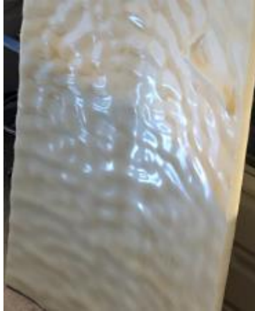
Figure 44. The wavy wall inside a High-Density Polyethylene Above-Ground Storage Tank
