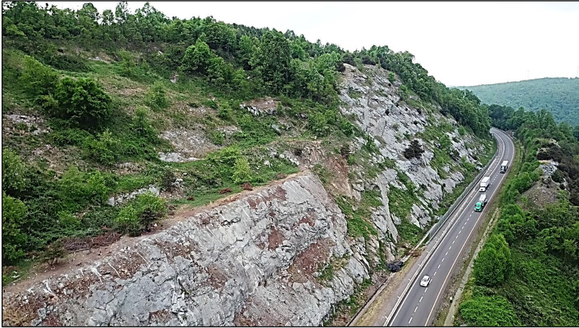
Figure 2. UAS photograph of Site #1 work area on I-77 at MP 5.4 southbound, looking north. Foreground shows slope after rock scaling in preparation for treatment with rockfall protection mesh. Distant slope is awaiting treatment.
