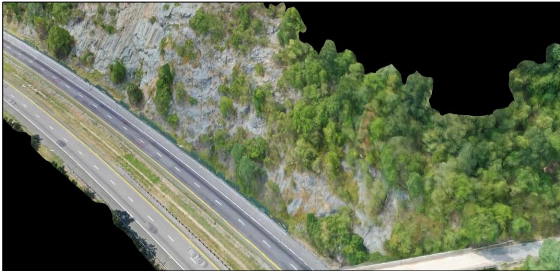
Figure 30. Site #5, Afton Mountain, I-64 Milepost 101. Farthest lanes are westbound. Densified point cloud with overlain triangle mesh, generated from UAS imagery using Pix4D Mapper .
