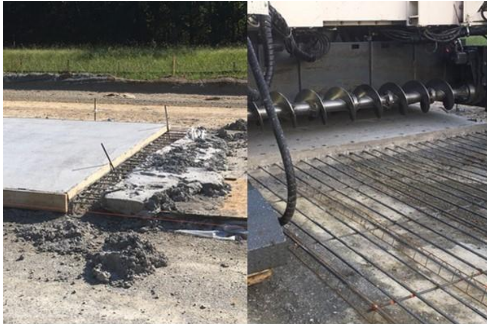
Figure 9. Construction Cold Joint With Regular Reinforcement
