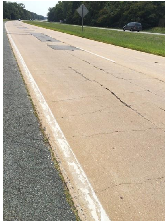
Figure 3. Surface Distresses on US 60W in September 2015
