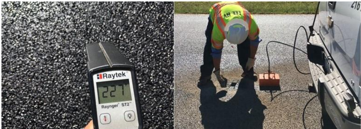
Figure 14. Checking SMA Laydown Temperature and Plug Extraction for Density Testing. SMA = stone matrix asphalt.
