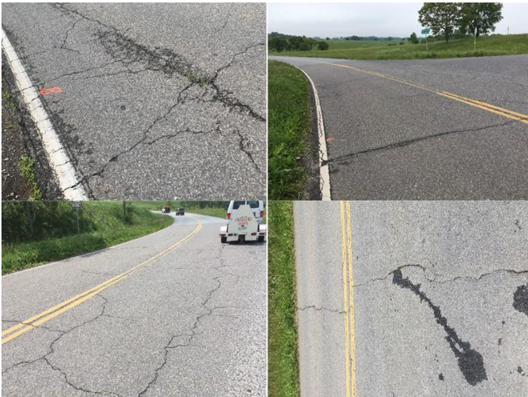
Figure 8. Pavement Surface Conditions at the Bedford County Test Site in 2017
