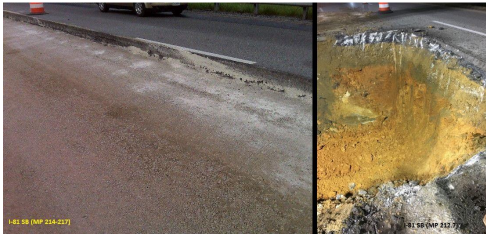
Figure 5. Examples of Base Layer Contamination on I-81 in Augusta County
