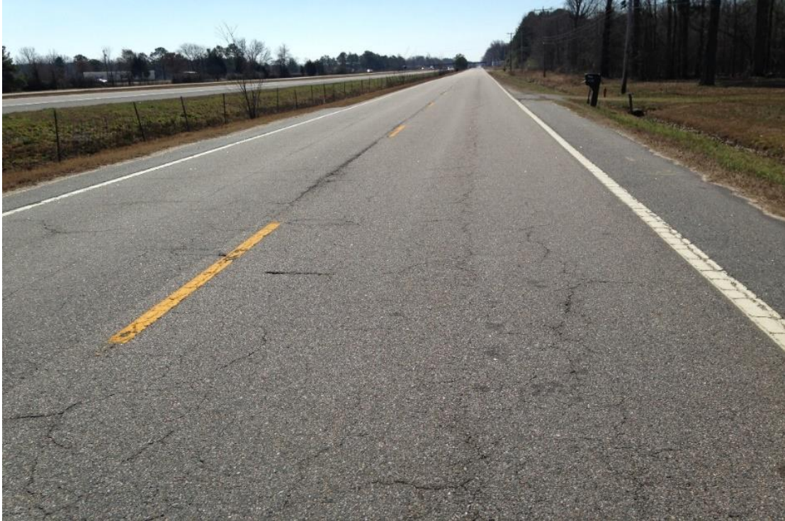
Figure 11. Section With Lower Amount of Cracking
