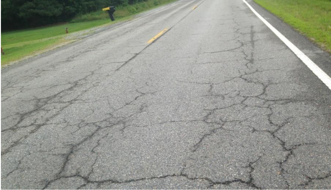
Figure 9. Section With Large Amount of Cracking
