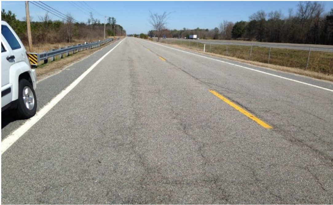
Figure 10. Section With Moderate Amount of Cracking
