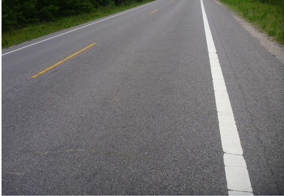
Figure 22. Modified Single Seal With Microsurfacing After 3 Years
