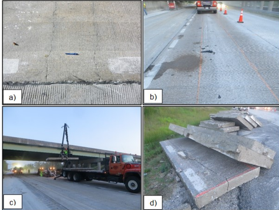
Figure 12. Patching on SR 288: a) area to be patched with closely spaced cracks; b) area selected for patching; c) old concrete slabs being removed; d) removed concrete slabs
