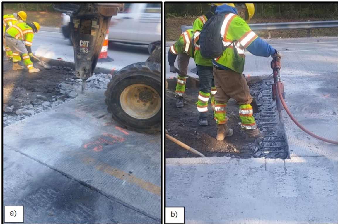
Figure 4. Hammer Breaking Concrete Next to Joint for Patching on I-85: a) larger hammer; b) smaller hammer
