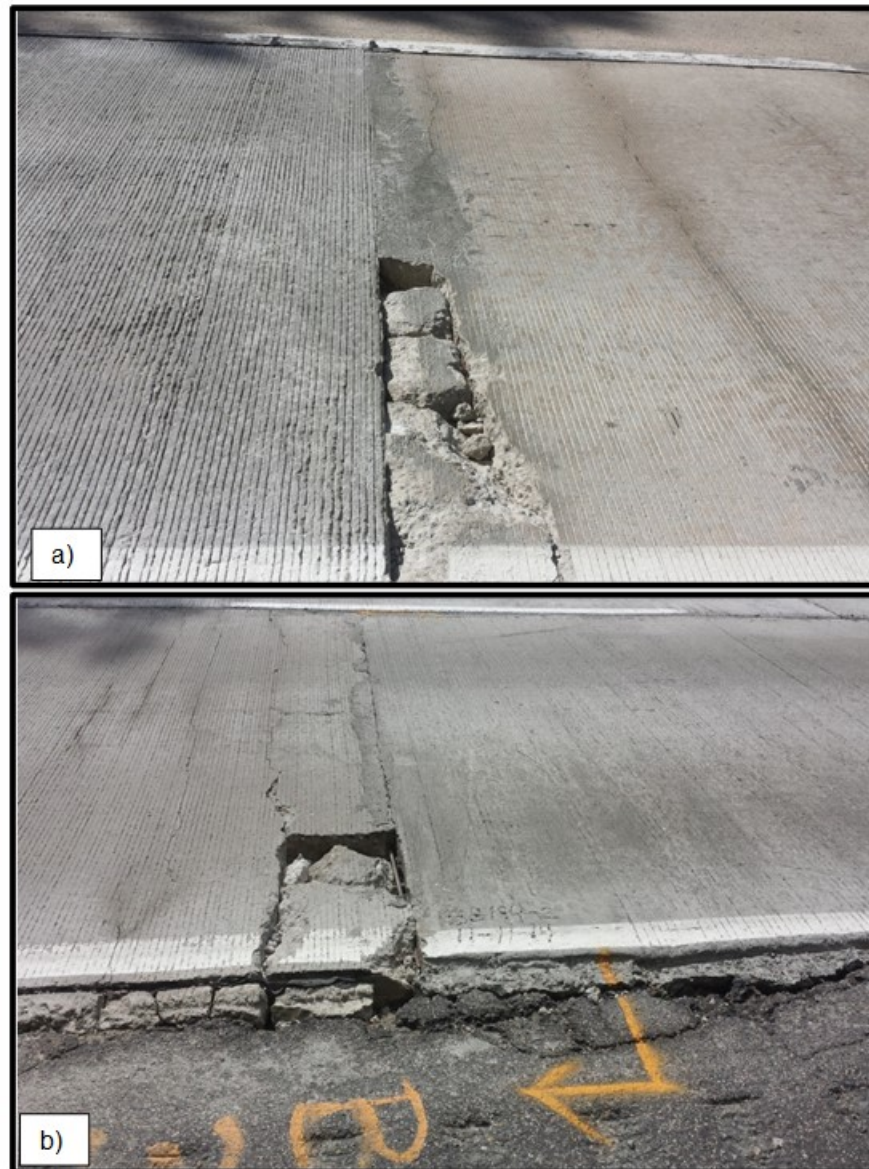
Figure 7. Joint Deterioration at Patches on I-85: a) new patch ( left ) next to 4-year-old patch ( right ); b) new patch ( right ) next to 4-year-old-patch ( left )
