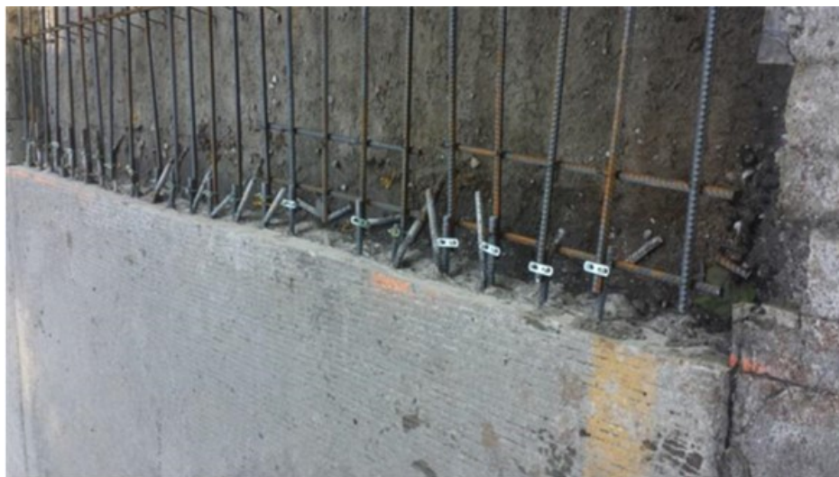
Figure 25. Short and Bent Reinforcing Bars on I-85 Patching
