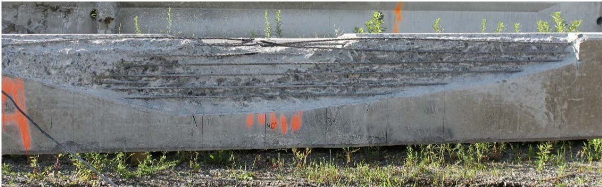
Figure 20. Damage Location for Test 4 Before Repair
