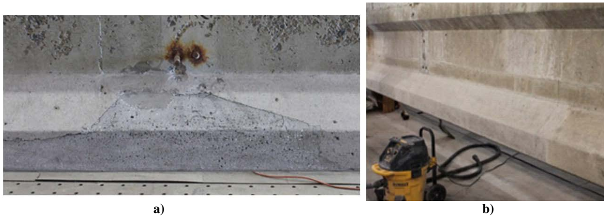
Figure 26. Repair Location a) After Formwork Removal and b) After FRCM Surface Preparation
