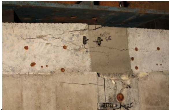
Figure 60. Compression Failure in the Composite Deck
