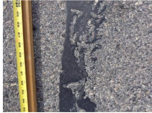
(b) Overband failure
