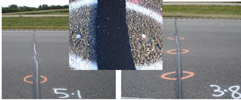
Figure 3. Crack Displacement Pins: Single-Point to Measure Only Right Wheel Path (left) and Three-Point to Measure Both Wheel Path and Middle of the Lane (right)
