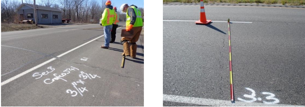
Figure 2. Initial Survey and Crack Numbering of a Test Section
