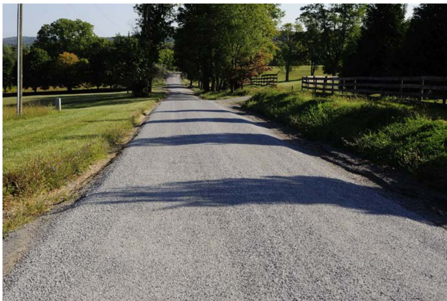
Figure 15. Repaired Cement-Stabilized Test Section on September 13, 2016
