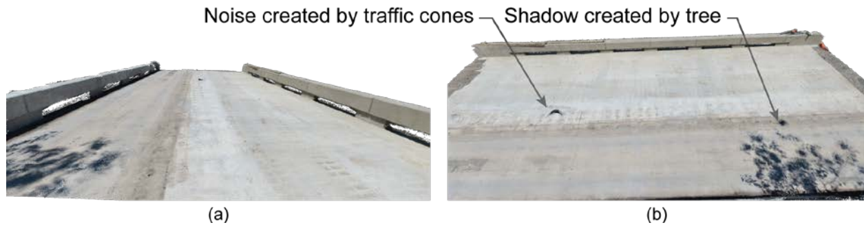
Figure 4. Example of a 3D Digital State Model of the Wolf Creek Bridge Deck During Construction: (a) Walking View Along the Bridge; and (b) Transverse-Looking View. This model is available online for viewing and downloading (Lama Salomon, 2016, 2017).
