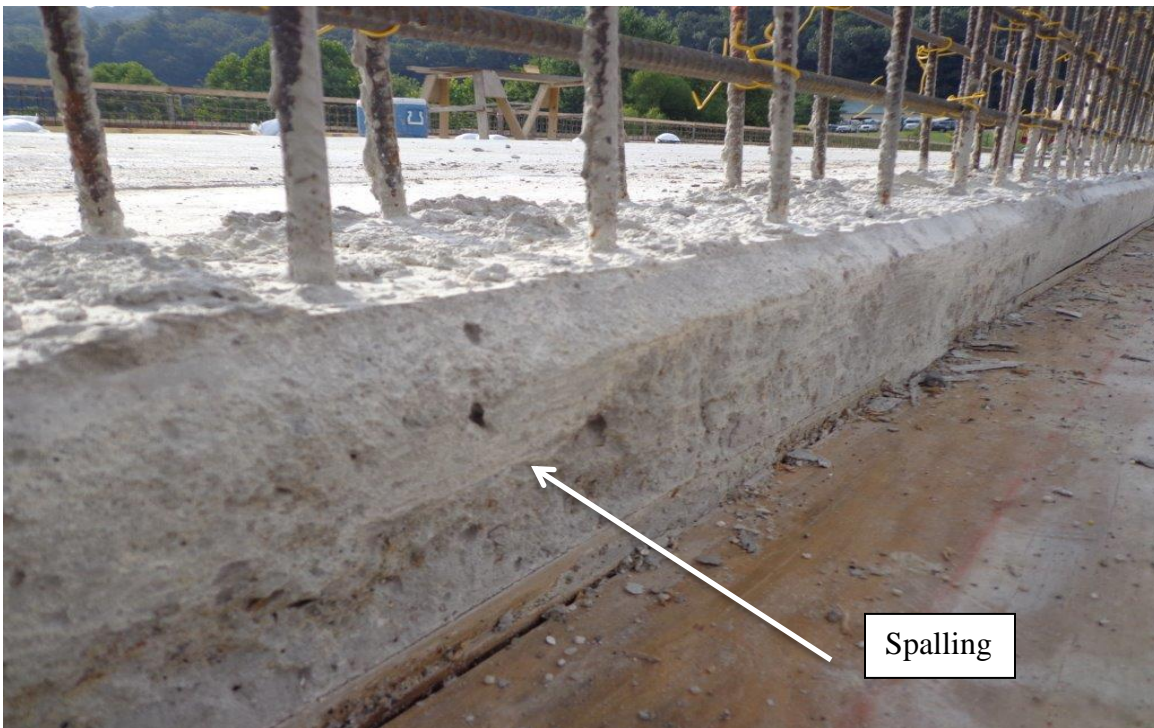
Figure 9. Spalling Along Edge of Route 613 Bridge During Form Removal
