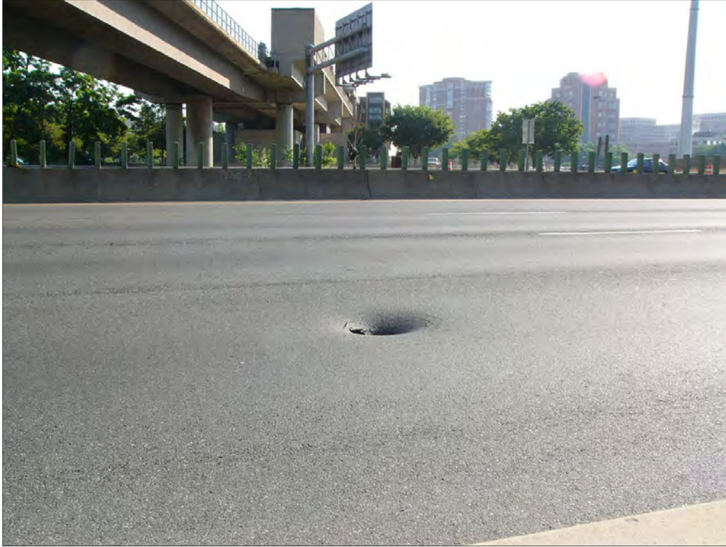
Figure 1. Roadway Subsidence After Trenchless Construction in Northern Virginia
