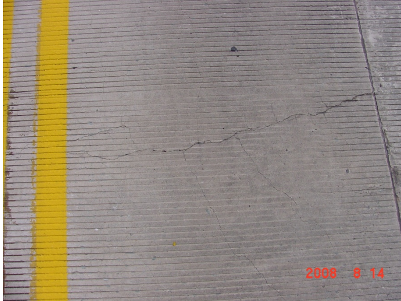
Figure 24. Deck Cracks (August 2008)
