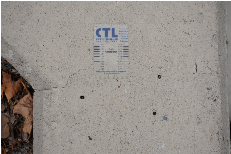
Figure 22. Wingwall Crack at Abutment B
