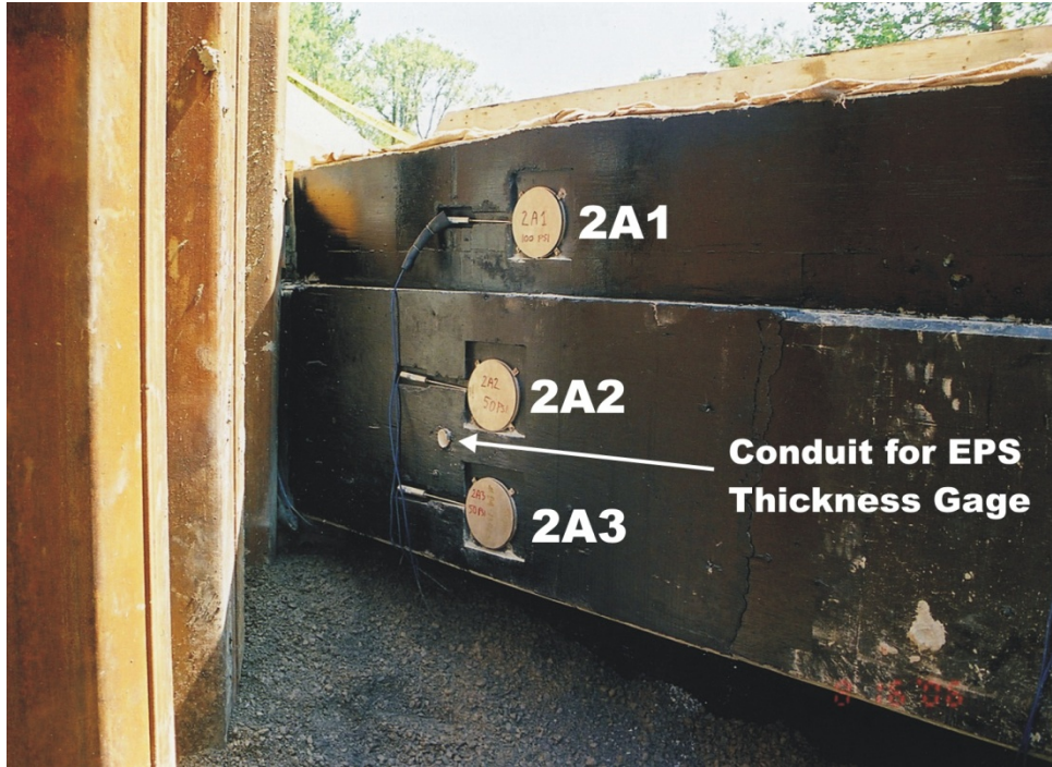
Figure 9. View of Some Pressure Cells at Abutment A
