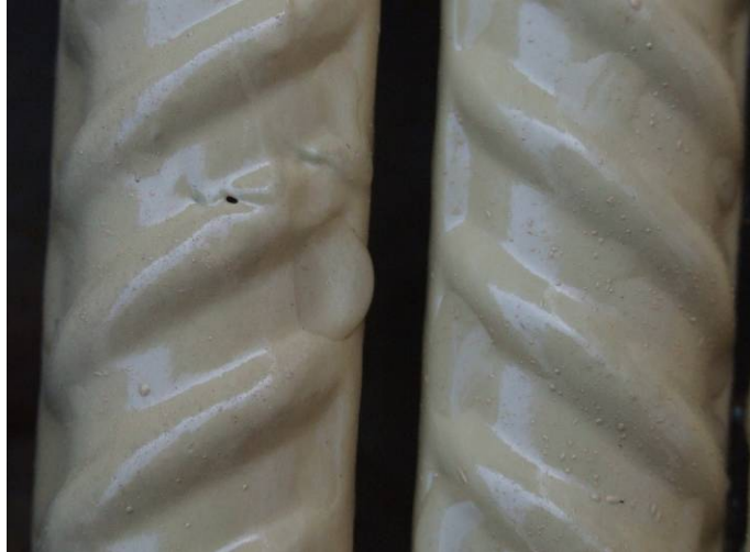
Figure 15. Pinhole in Zbar coating.
