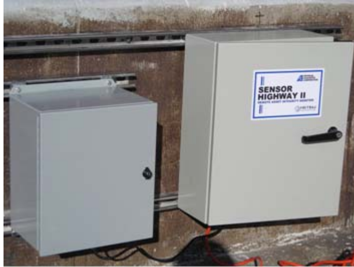
Figure 6. Sensor Highway II DAQ System and Battery Backup
