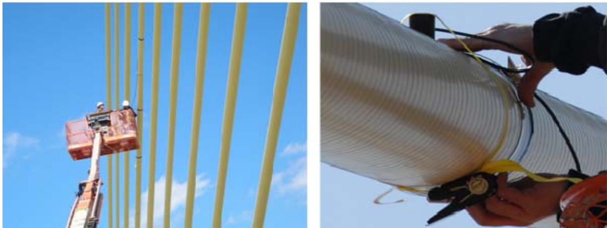
Figure 2. Left , Overview of AE Sensor Installation at Selected Locations on Cable 10; Right , Close-Up of Installation of Single AE Sensor
