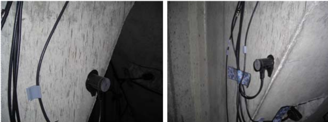
Figure 4. Typical Photographs of Sensors Affixed on Concrete Walls of Cable Saddle
