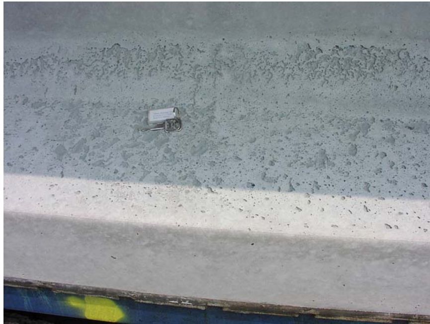
Figure 2. Bugholes on Web and Top of Bottom Flange
