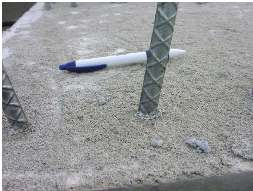
Figure 3. Frothy Look on Top in Concrete With High Flow Rate
