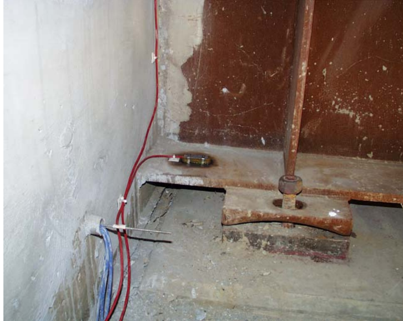
Figure 6. EPS Rod and Lower Flange Strain Gage
