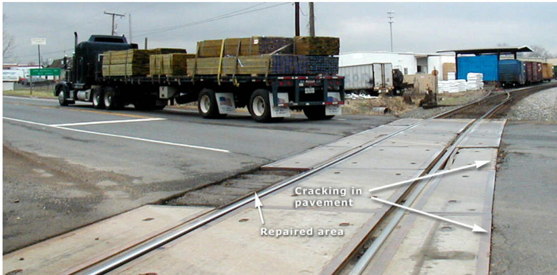
Figure 5. Concrete Panel Crossing Repaired with Hot-Mix Asphalt and Deterioration of Approach Pavement.
