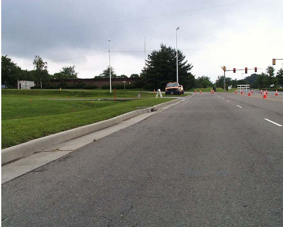
Figure 2. Displaced Curb and Gutter Above Culvert Pipe, Old Airport Road.
