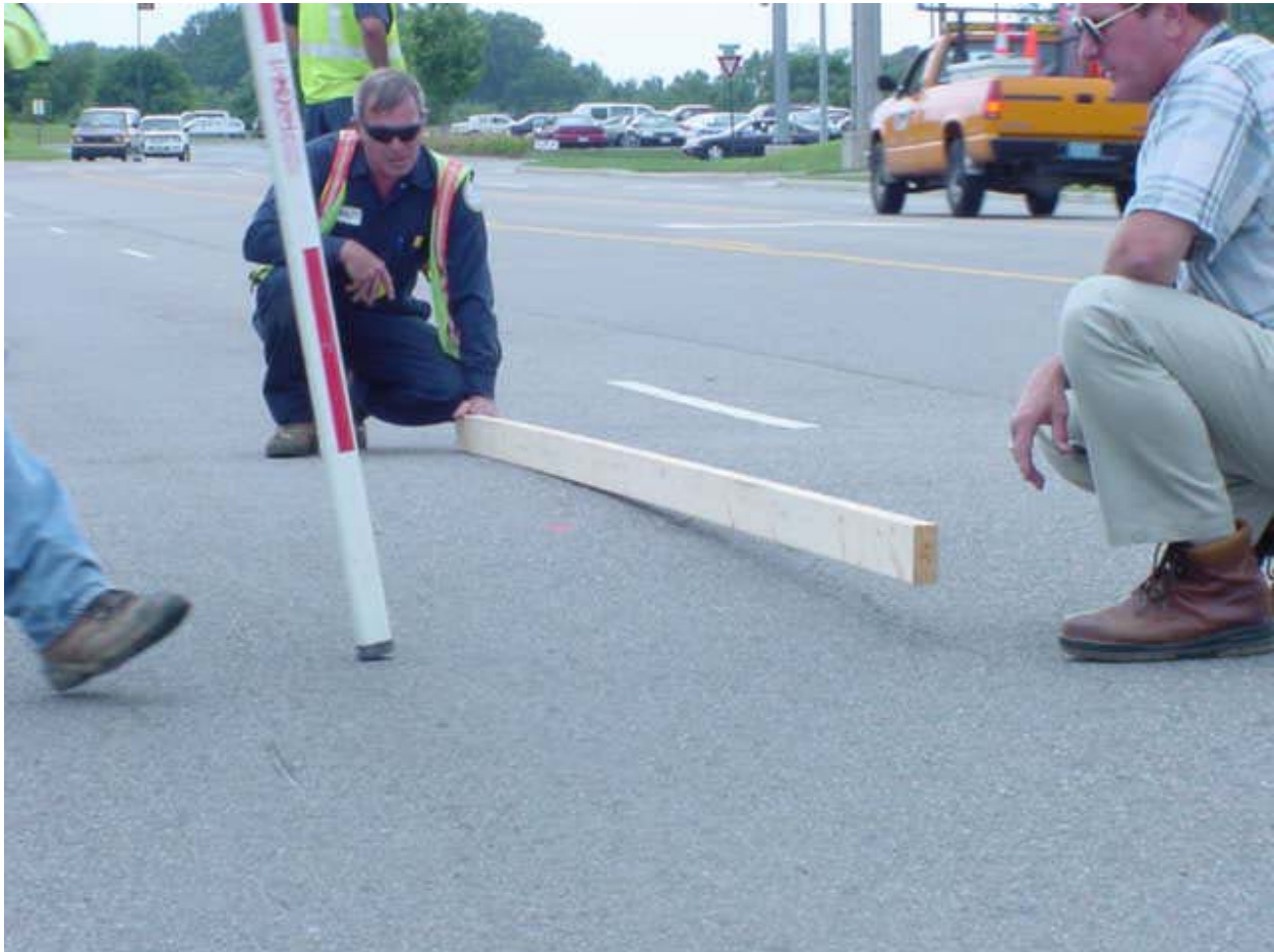
Figure 1. Pavement Surface Distortion, Old Airport Road Near Coronet Drive.
