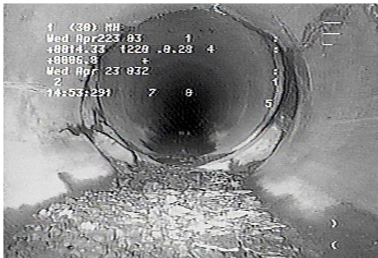
Figure 3. Video Image of Damaged Culvert Pipe Beneath Heaved Pavement.
