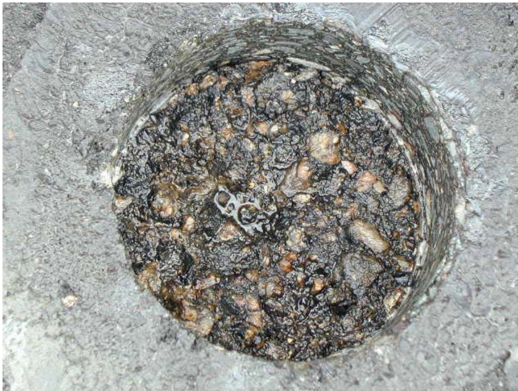
Figure 9. Typical Moisture Damage in Underlying Layer (Core 2-8)
