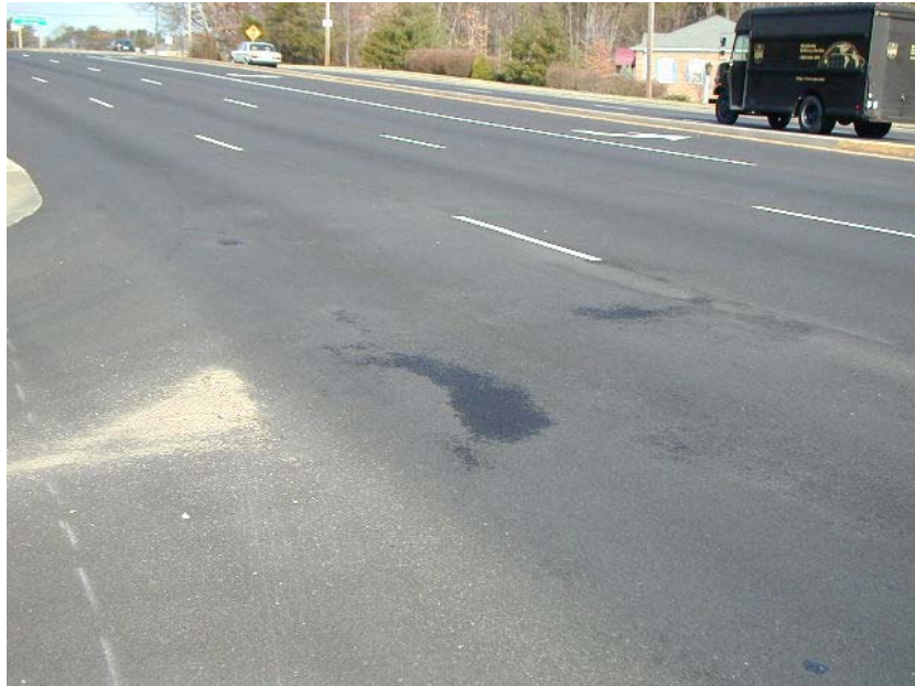
Figure 2. Wet Spot on Old Bridge Road Near Wood Hollow Drive
