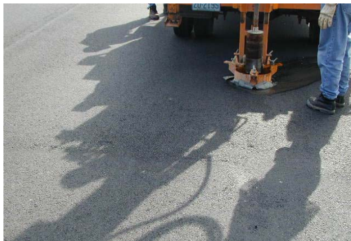
Figure 5. Segregation at Transverse Cold Joint
