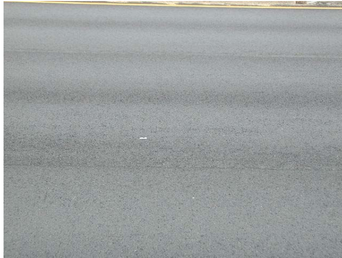
Figure 4. Centerline and Longitudinal Joint Segregation
