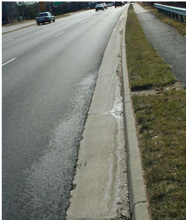
Figure 3. Wet Area at Edge of Pavement
