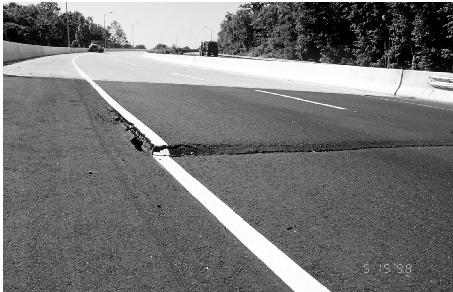
Figure 4. Approach Slab Distress Attributable to Foundation Soil Settlement (Rte. 10 westbound lane over the Appomattox River)
