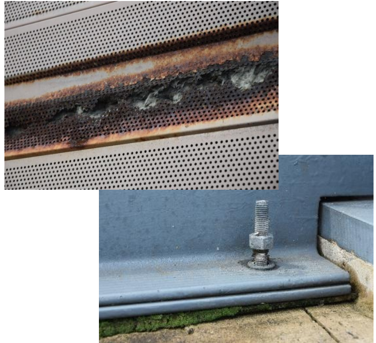
Top: Heavily corroded metal noise barrier panel. Bottom: Fractured anchor bolt due to corrosion.
